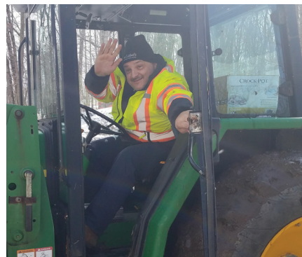
Past President Angelo Porecca preparing the land for the chapter's new home base at Community Park. They are getting ready for Belle Italia in September.
